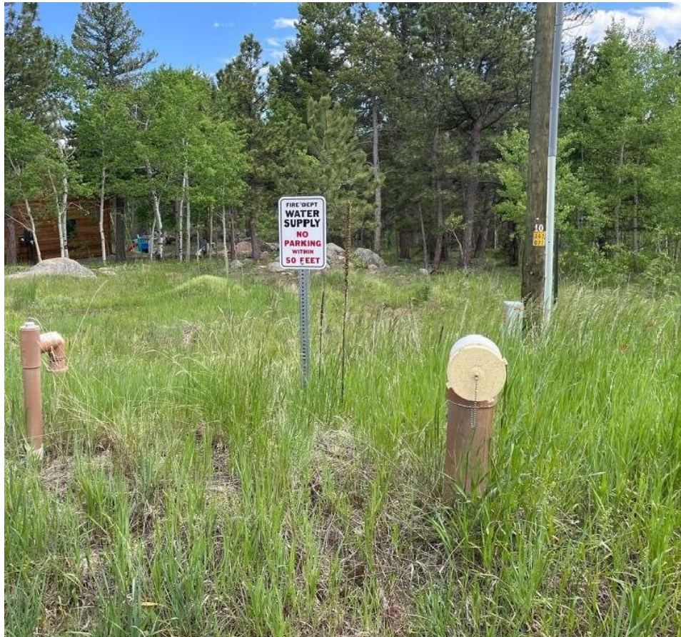
Figure 33: Local cistern. Photo credit: The Ember Alliance
